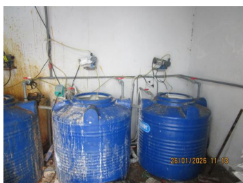
Chemical tanks at wastewater treatment system.jpg
